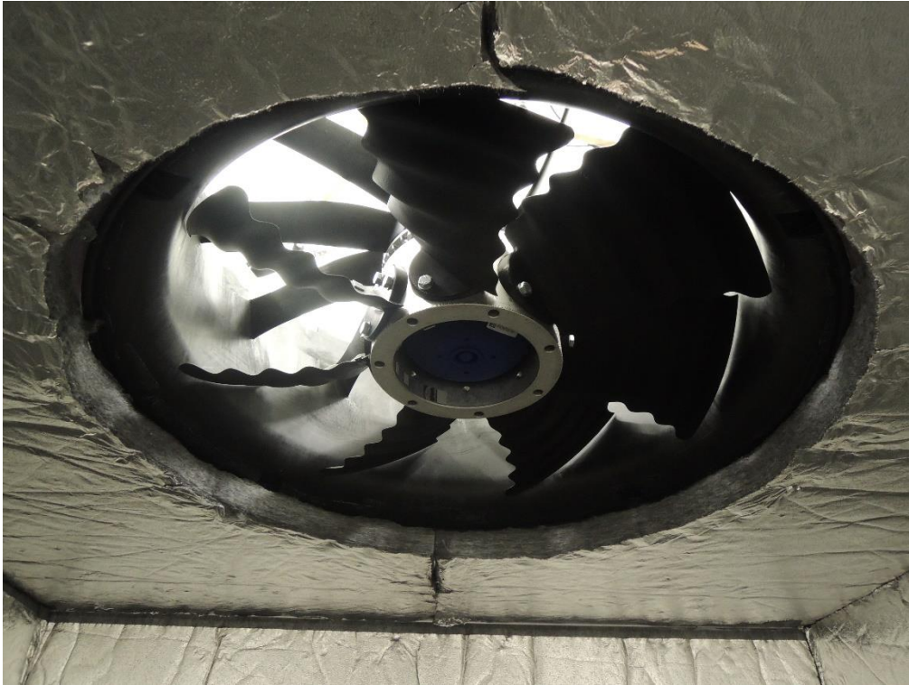
Figure 5.8: GreenHP with mounted sound absorbers (inner view towards the fan, detail)
